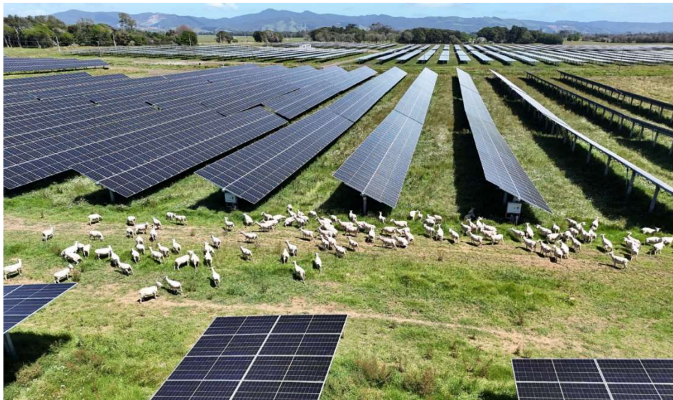
Figure 2. A utility-scale 33 MW DC single-axis tracker (2P) solar array (60,000 modules at 540 W each) covering 200 acres of farmland in Kaitiā, Northland, New Zealand. Pivot point: 6.6 ft above the ground, posts extend up to 14 ft underground. Completed in November, 2023.
