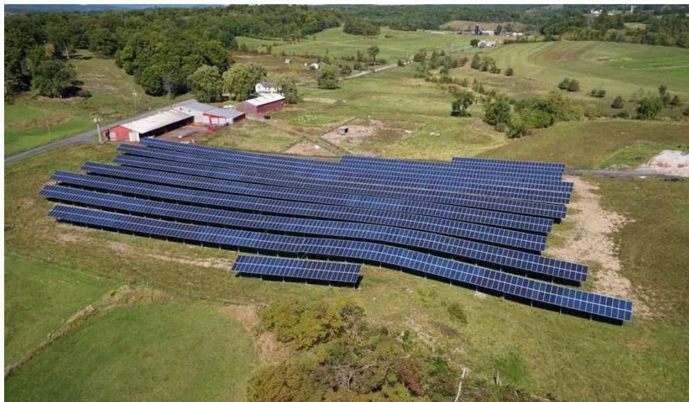
Figure 1. A 500 kW fixed-tilt (2P) solar array (2,300 modules) covering almost 5 acres of a Benson, VT farm allows cattle to graze in areas shaded by solar panels. Tilt angle: 30°, minimum clearance: 8 ft, posts extend up to 12 ft underground. Completed in June, 2016.
