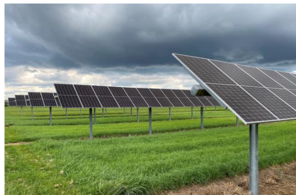
Figure 2: Single-axis trackers at Snyder Farm in Pittstown, NJ.
