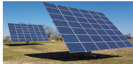
Figure 4: Dual-axis tracking array. Image credit: https://www.solarcentex.com/dual-axis-trackers/ ; no endorsement implied.
