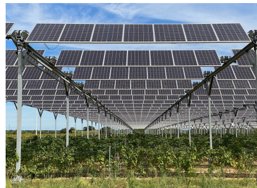
Figure 5: Raised single-axis tracking array. Image credit: https://sunagri.fr/en/solar-panels-help-french-winemaker-hold-off-climate-change/ ; no endorsement implied.
